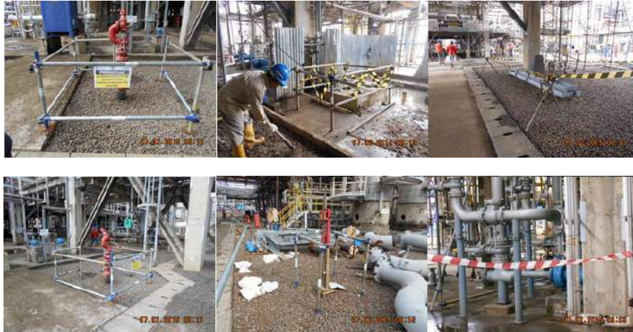
Figure 4. 3 Safety Barricade Example on CAP
